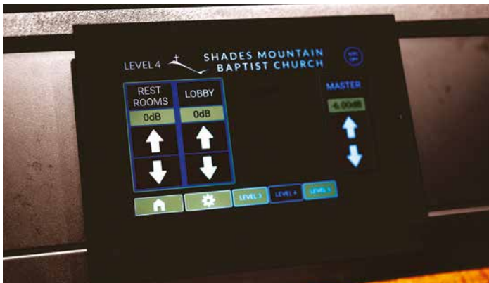
Q-Sys control is offered via touchscreens
